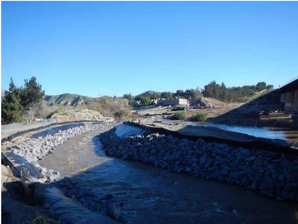
Photograph 2: View of the Santa Ana River diversion channel located immediately upstream of the BNSF railroad, facing northeast.
